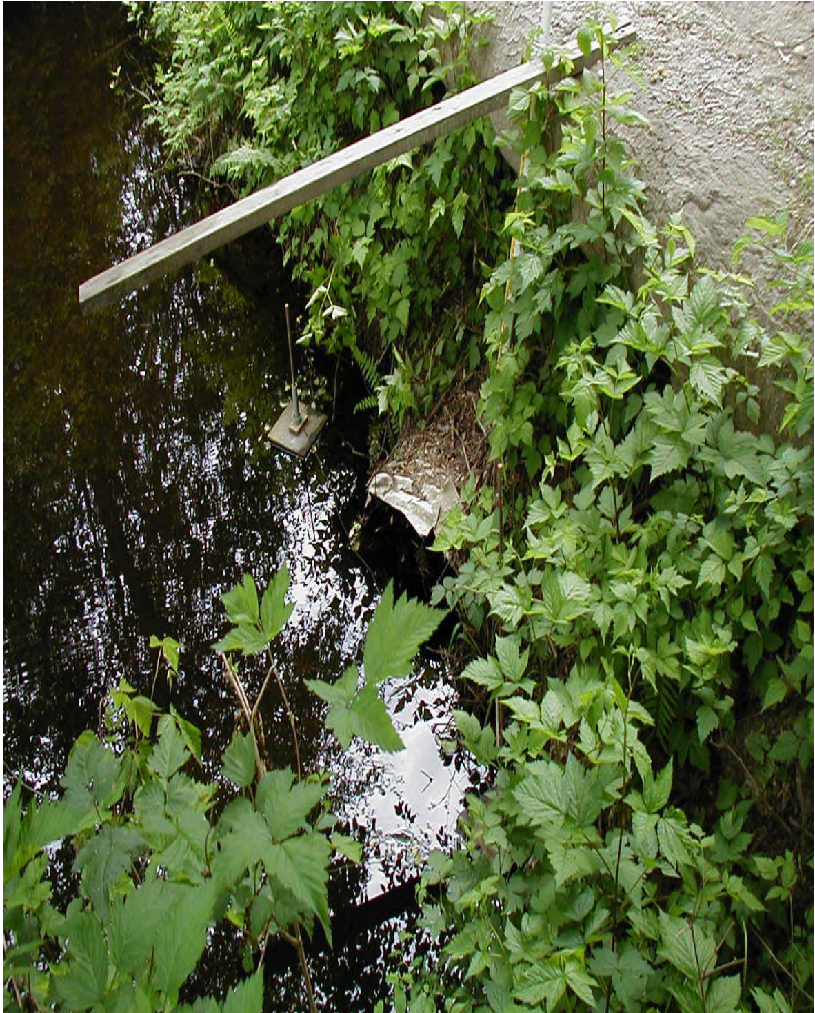
Undersized culvert under 228 th and blocked Bear Creek stream flow
