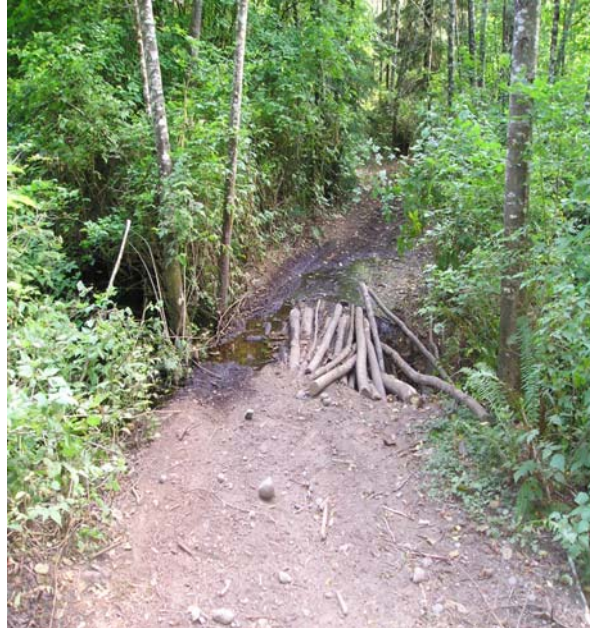
Section IV trail crossing Bear Creek Tributary, June,2003; crushed culvert and logs that were blocking stream flow were removed July, 2003.
