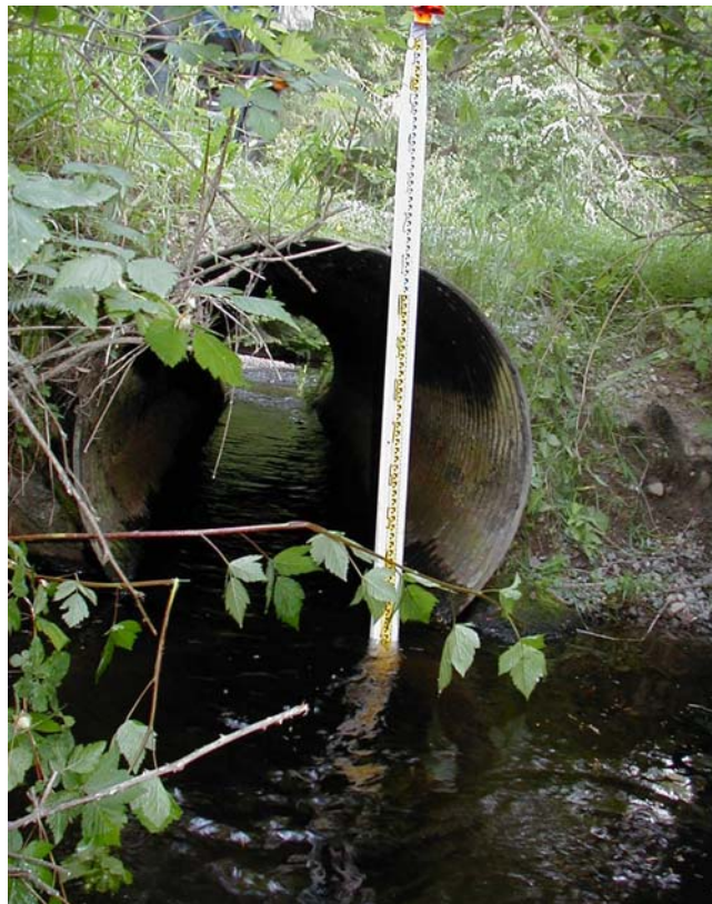
Bear Creek flowing through an undersized culvert under E-W easement road
