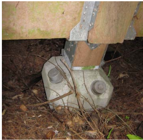
The pier block here was placed more superficially above these tree roots.
